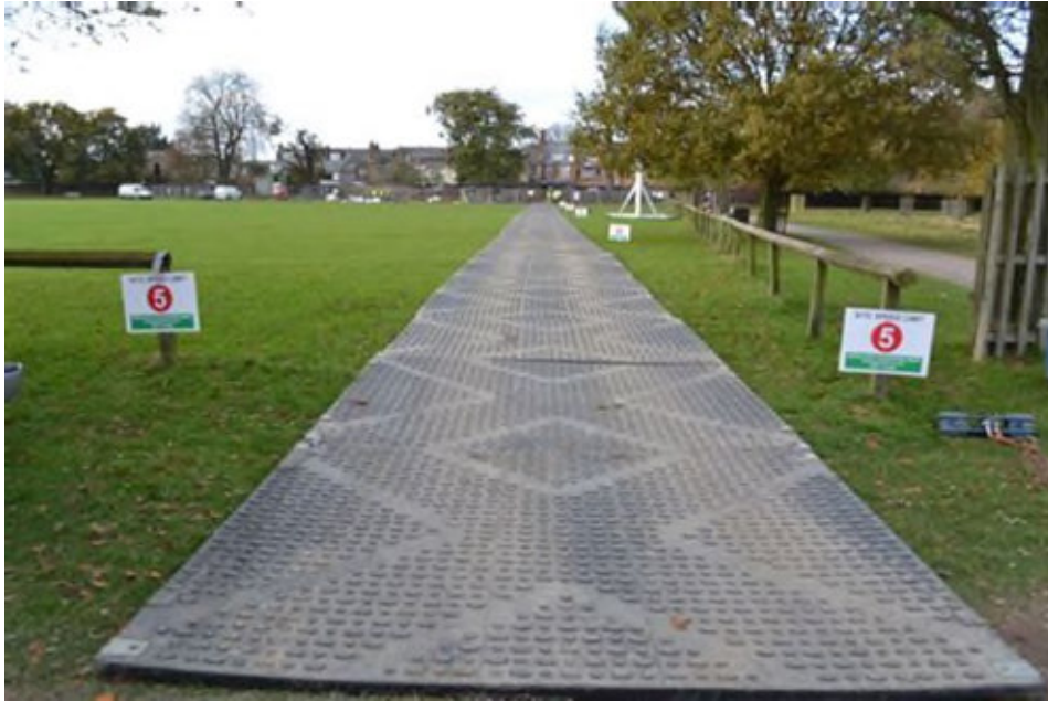
Figure 1.7 – Typical temporary interlocking matting/panels to protect the ground during access and egress (To be used through the scheduled monument to avoid ground damage)
